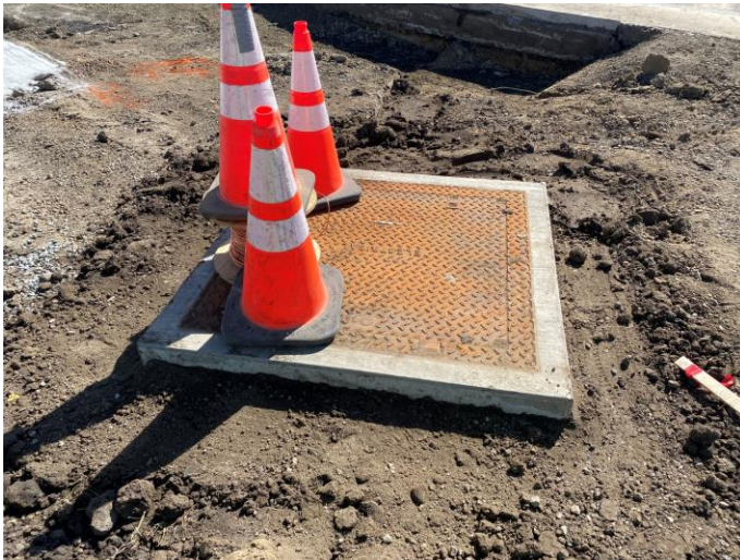
Electrical pullbox installed
