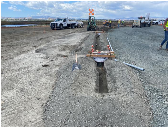
Electrical trench along Taxiway H curve
