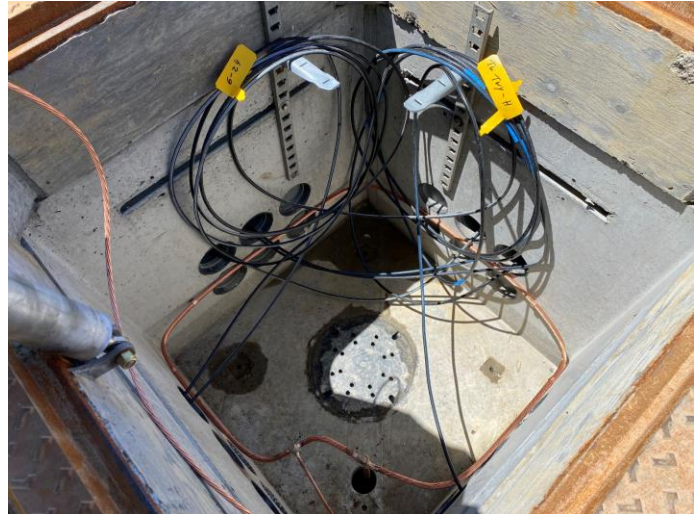
Cable and grounding in pull box
