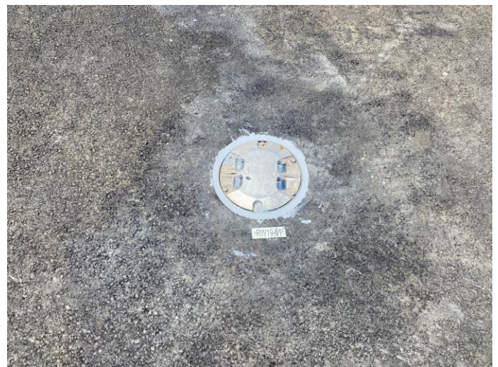
In-pavement runway light installed
